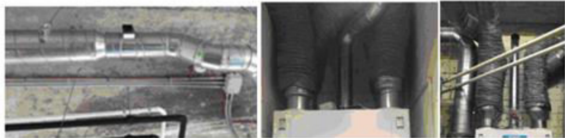
Fig 9. Ventilation system equipment [from personal archive]
