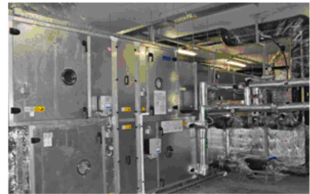
Fig 6. Example of central air handling unit [from personal archive]
