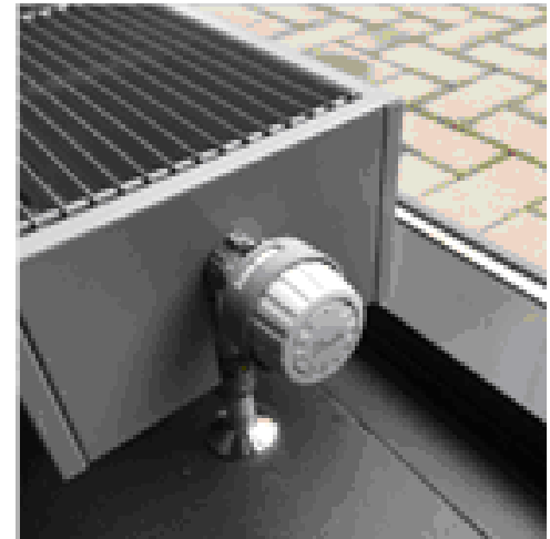
Fig 16. Heating systems devices [from personal archive]
